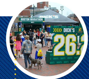
Battery-powered generators at events
